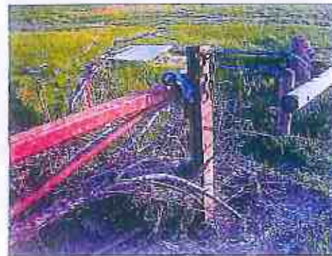
Flood damaged infrastructure
