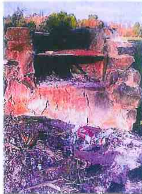
Poorly designed and maintained facilities
