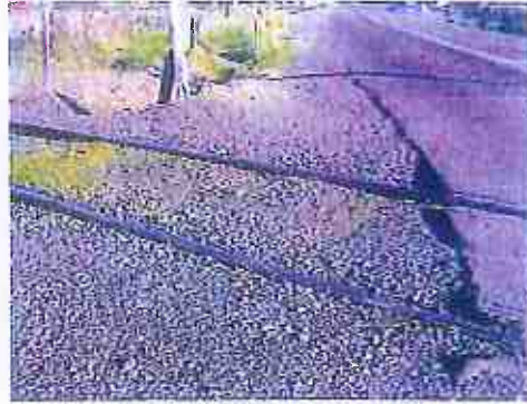
Raised railway lines and uneven surfaces
