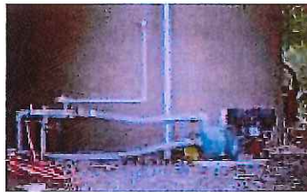
Figure 7 - Protect above ground pipes and pumps
