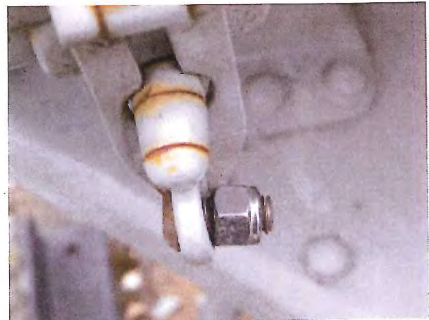
Fig 4 Minor surface corrosion on fittings
