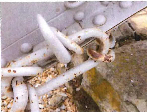
Fig 3 Minor surface corrosion on fittings
