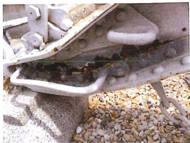
Fig 6 Badly corroded end section frame
