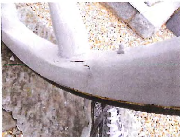
Fig 11 Deterioration of wooden rim
