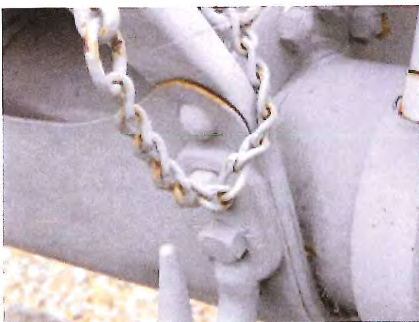
Fig 5 Minor surface corrosion on fittings
