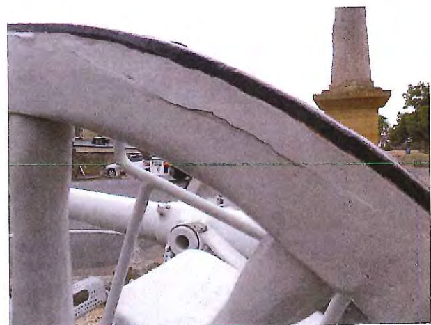
Fig 12 Major crack – proper left wheel
