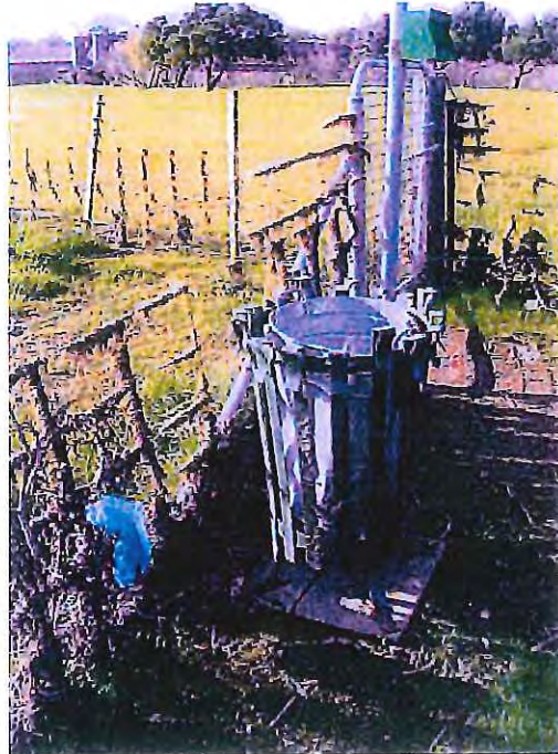
Fences prone to collecting flood debris
