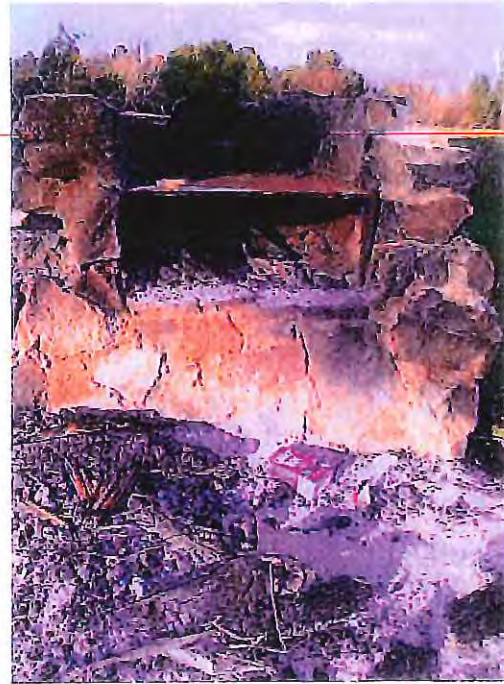
Poorly designed and maintained facilities
