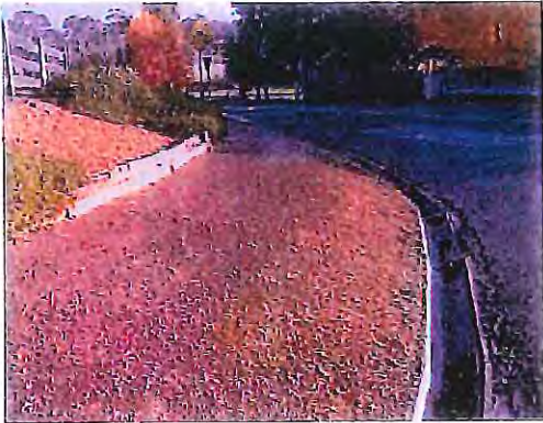
Dangerously cambered path and spoon drain
