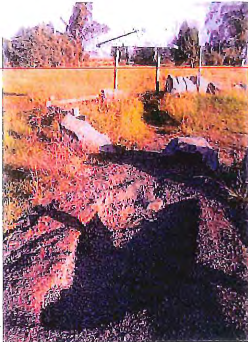
Unrepaired flood damage to paths
