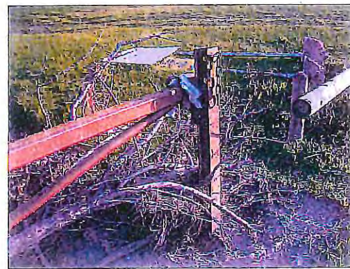
Flood damaged infrastructure
