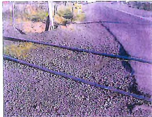
Raised railway lines and uneven surfaces
