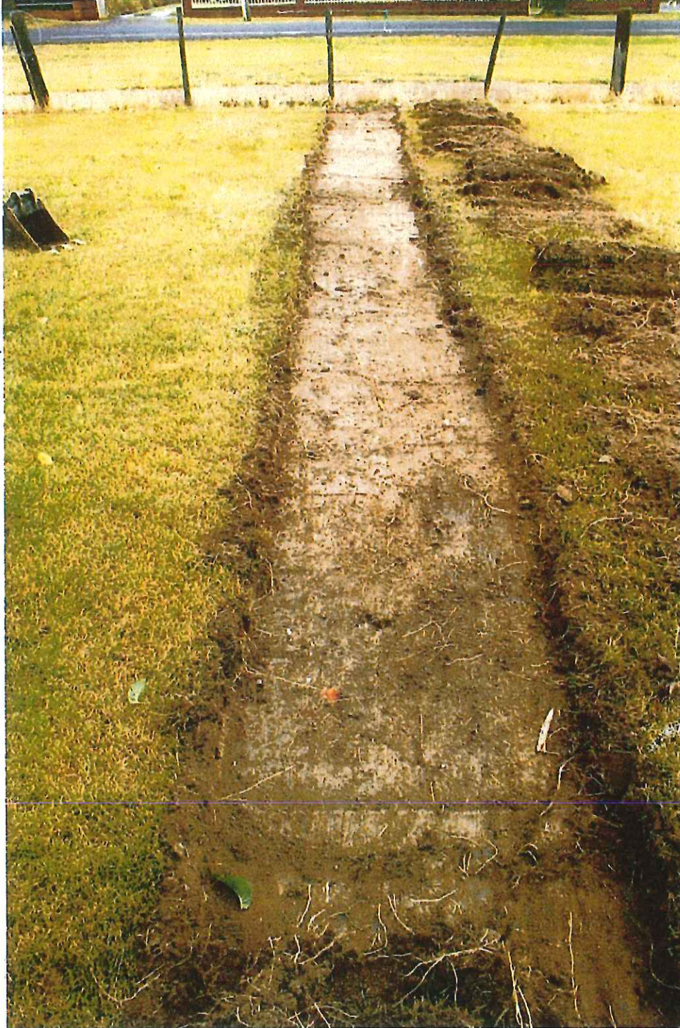
Figure 3.8 – The proposed service trench to the existing Sunday School building following removal of topsoil. Further excavation of this line also yielded sterile ground.
