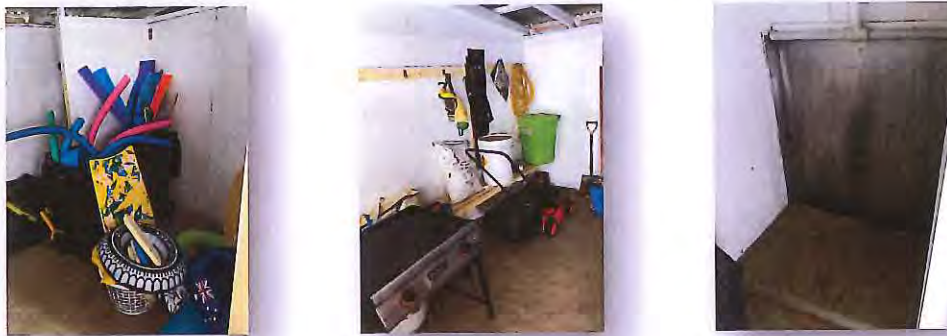
Figure 8 – Existing amenities are outdated and currently used for storage of most maintenance and safety equipment.
