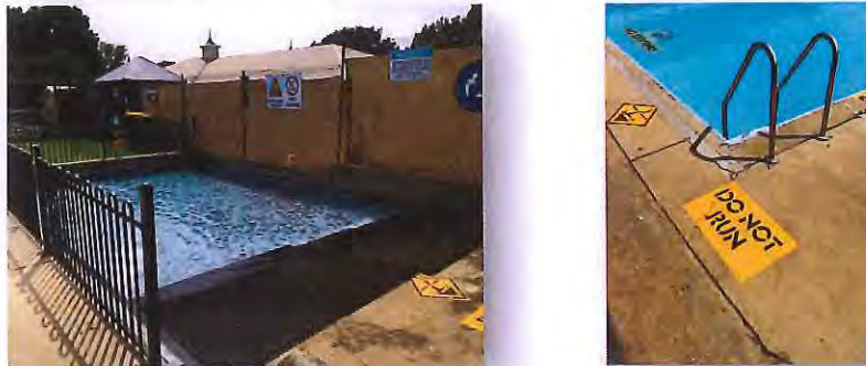
Figure 6 – Toddler pool surfaces, balustrades and pool concourse require upgrading to safer options.
