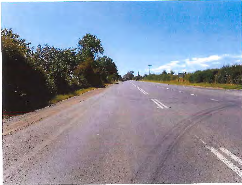
Photograph 6.1: View of sealed and gravel sections on northbound section of Hobart Road
