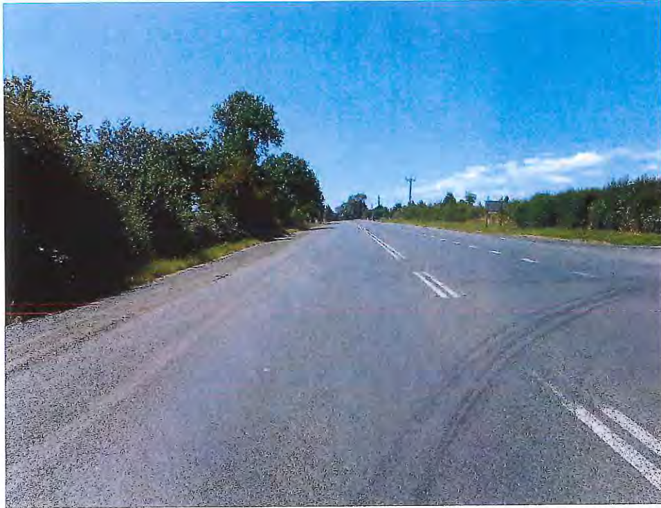
Photograph 6.1: View of sealed and gravel sections on northbound section of Hobart Road
