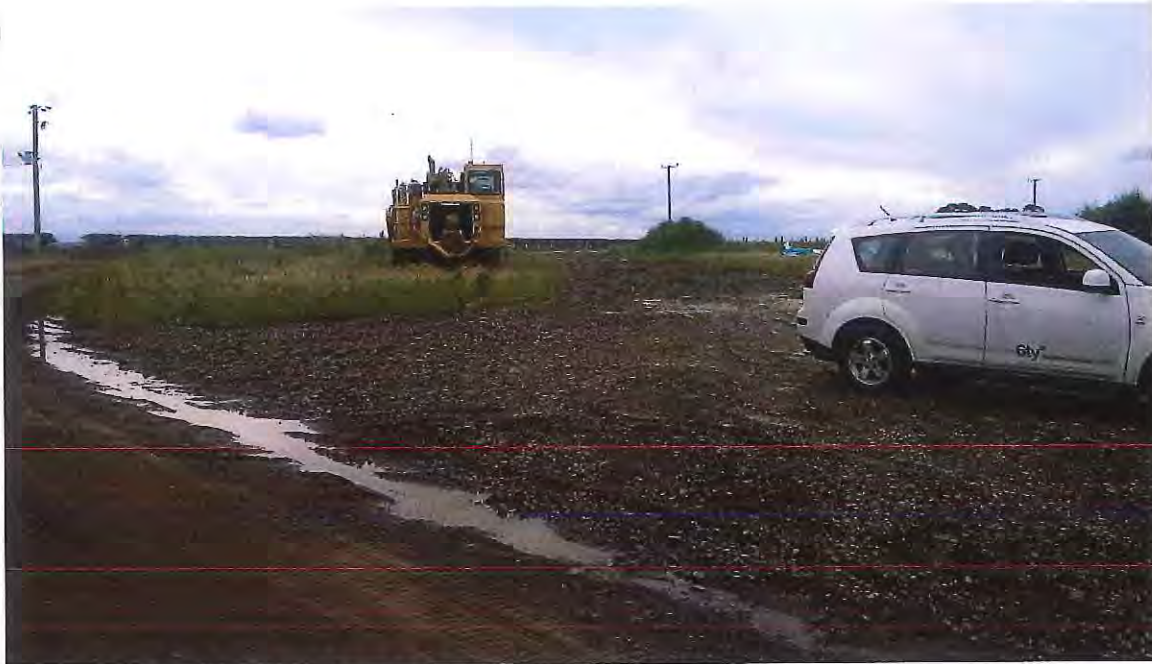
Image 5 - The road bend and the two driveways.
