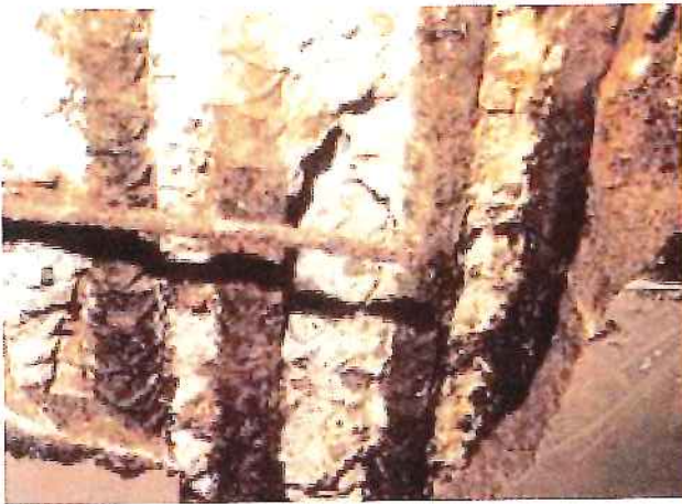
Fig. 6-16. The damage to this concrete parking structure resulted from chloride-induced corrosion of steel reinforcement. (50051)
