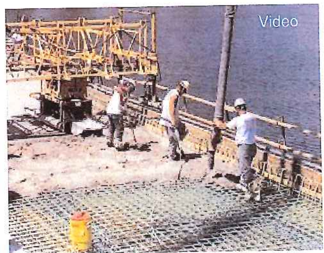
Fig. 6-6. Low water to cement ratio concrete with low chloride permeability—easily made with high-range water reducers—is ideal for bridge decks. (69924)
