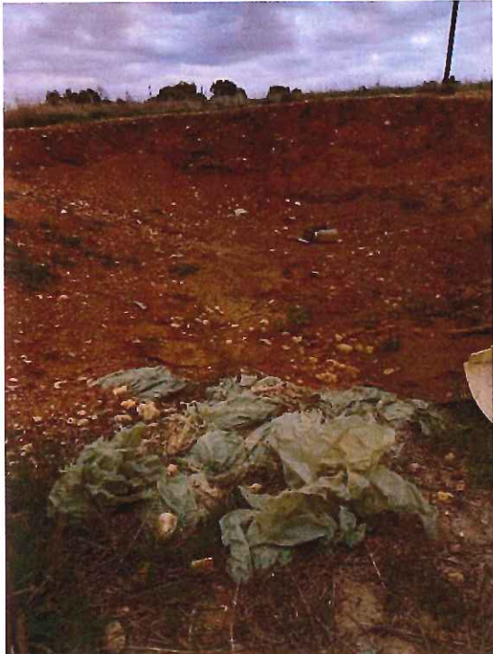
Typical debris observed
