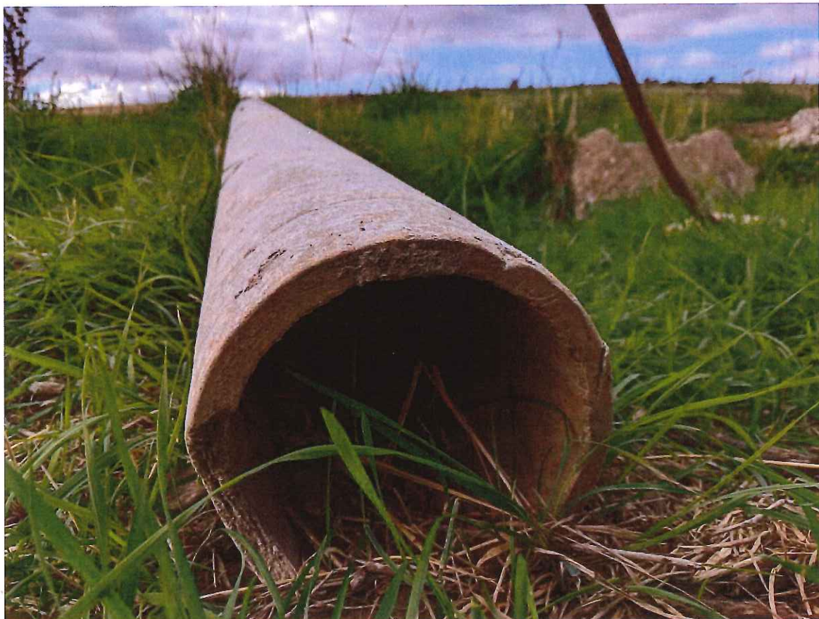
Observed disused potential asbestos containing water pipe
