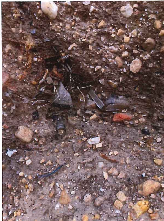
Exposed fill with concrete, brick and glass
