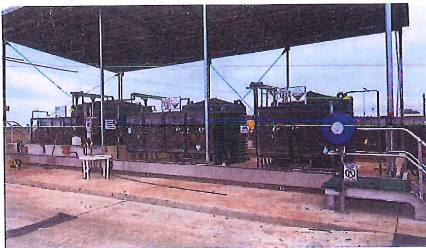
Figure 13 - Chemical storage and dosing facility at Kingaroy
