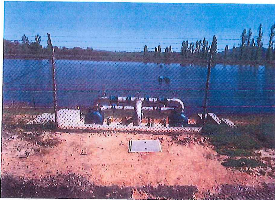
Figure 8 - Typical Lagoon return pumps
