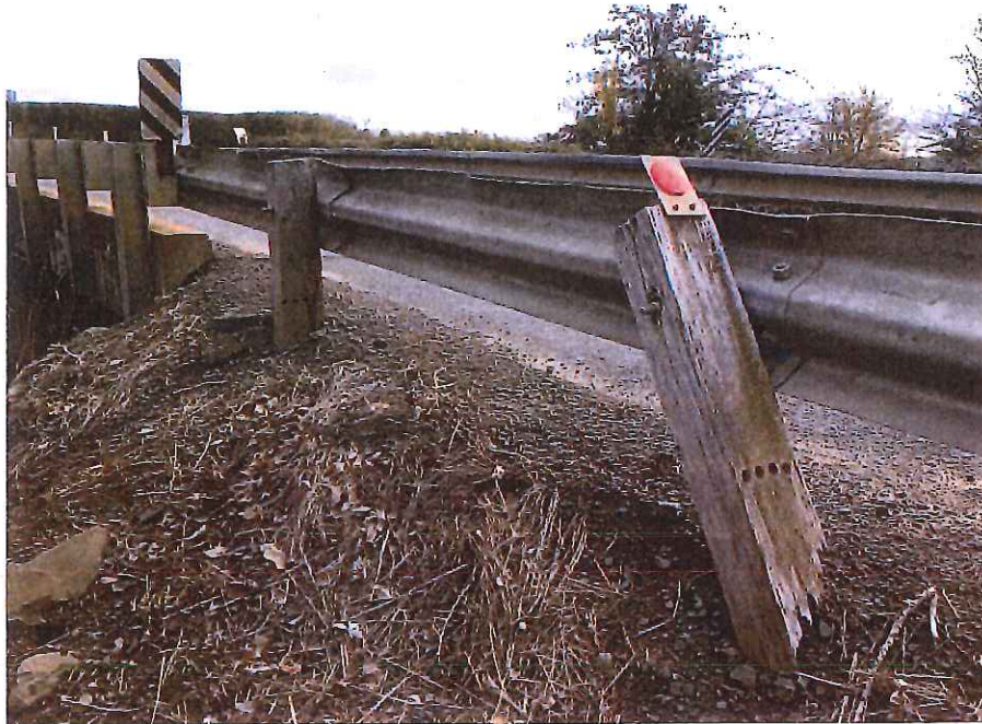
Photo 5 – View of poor condition barriers
