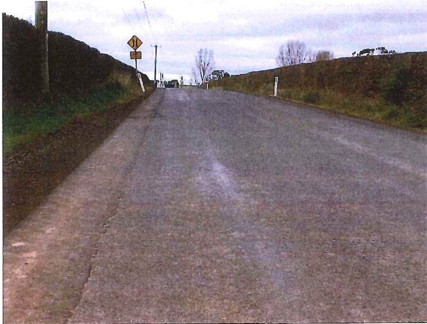
Photo 2 – Lack of Bridge visibility on western approach
