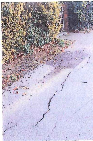
Footpath cracking and repaired sinkhole Wellington St.
