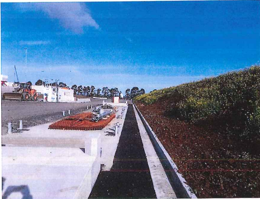
Figure 3- site looking east, batch plant on the left and landscaped mound on the right.
