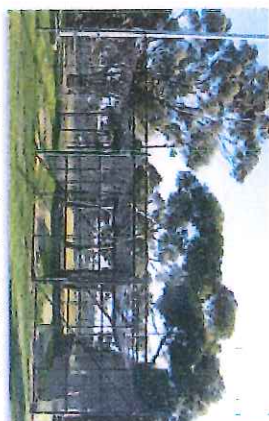
Example of poor quality and unsafe infill materials Image courtesy of InsideEDGE Sport and Leisure Planning
