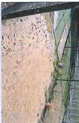
Example of poor quality and unsafe infill materials Image courtesy of InsideEDGE Sport and Leisure Planning
