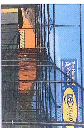
Example of damage to a flat roof net design Image courtesy of InsideEDGE Sport and Leisure Planning
