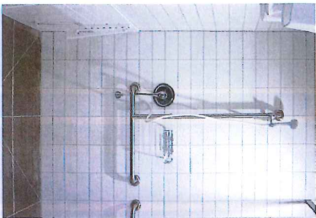
Example of an accessible shower facility Image courtesy of JMA Architects
