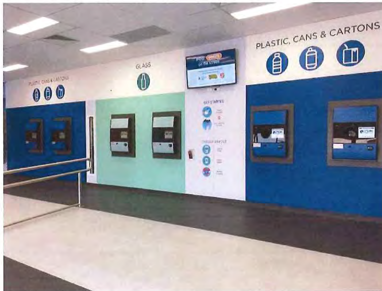
Figure 5: Small RVMs installed along wall, forming a mini recycling centre Credit: https://www.perthnow.com.au/community-news/stirling-times/was-containers-for-change-deposit-scheme-officially-up-and-running-c-1351180
