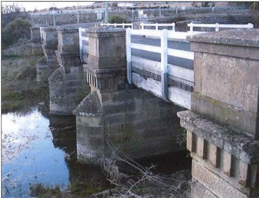
PLATE 2 VIEW OF THE DOWNSTREAM SIDE OF THE BRIDGE TOWARD THE HIGHWAY
