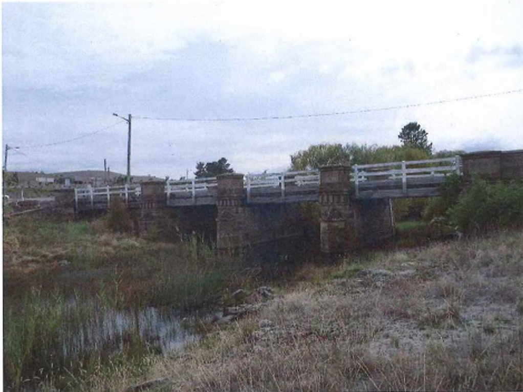
Figure 2: The Blackman River Bridge view of the upstream facade, looking to the north east (2015).
