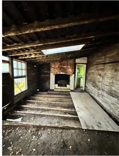
View of back wall from point 3, showing severe dilapidation, and structural failure of the rear wall. Photo taken 18th April, post lining removal.
