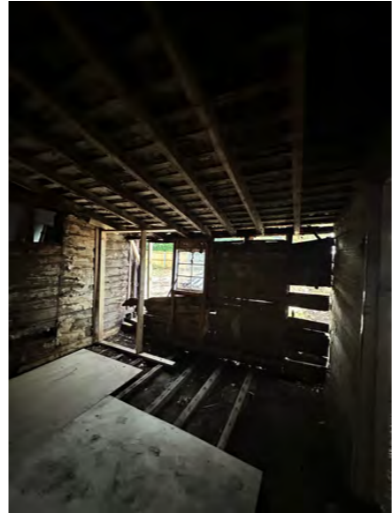
View of back wall from point 1, showing severe dilapidation, and structural wall failure of the rear wall. Photo taken 18th April, post lining removal.
