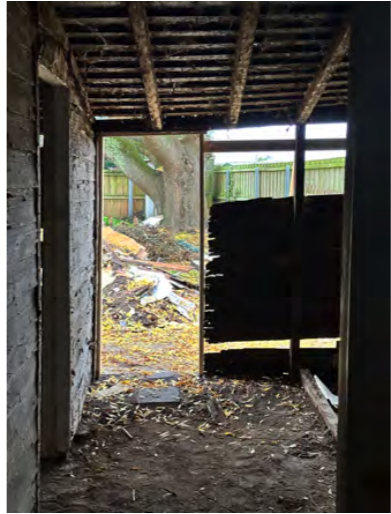
View of back wall from point 2, showing severe dilapidation, and structural failure of the rear wall. Photo taken 18th April, post lining removal.
