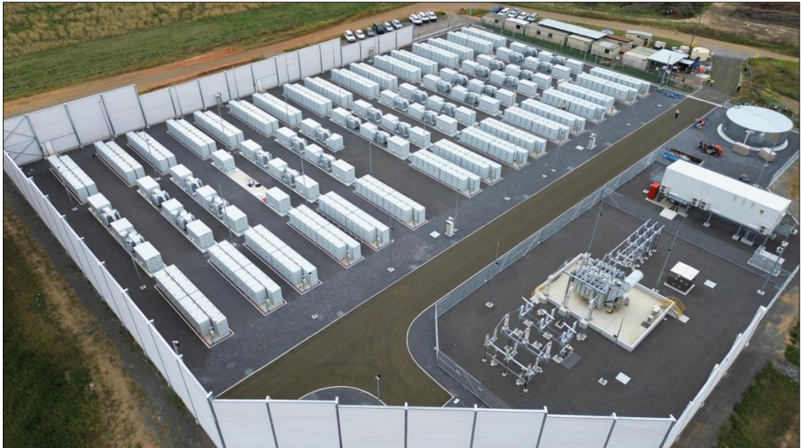
Figure 16: Capital Battery showing tall thin lightning protection masts
