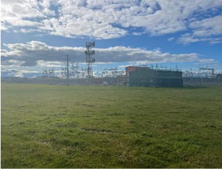
Photo 4: Portion of the battery storage location shown in the foreground of the photo looking north-east towards the TasNetworks Palmerston Substation.
