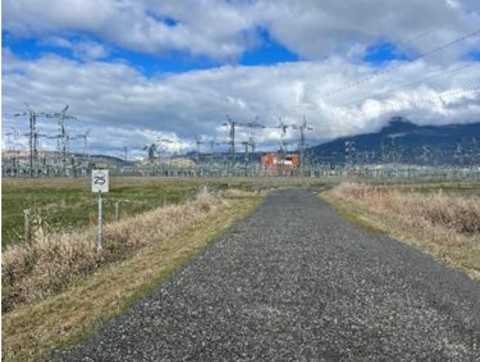
Photo 2: TasNetworks Palmerston Substation, looking south from the internal road.
