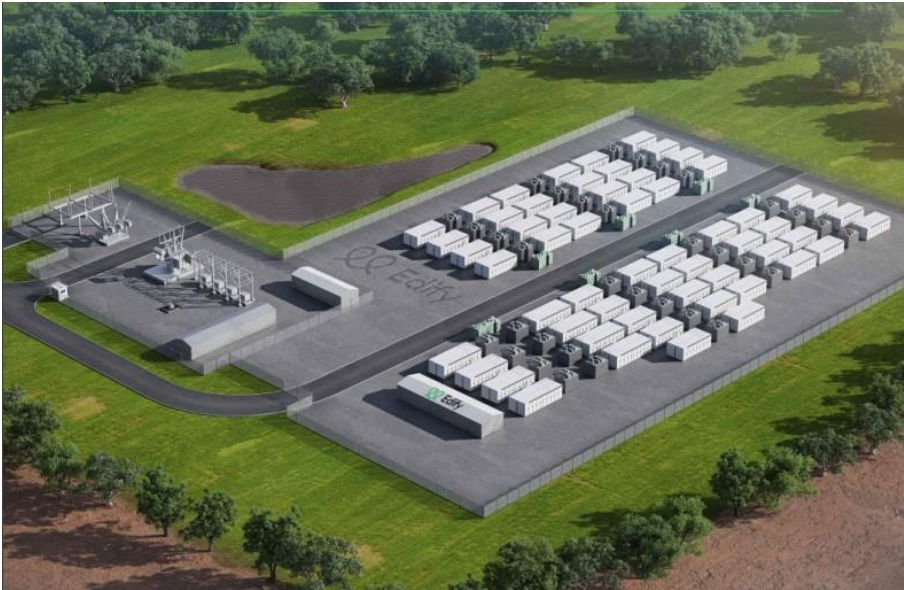
Figure 1 Typical Large scale Battery Energy Storage facility layout - Darlington Point NSW. Source Edify: Darlington Point & Riverina Battery
