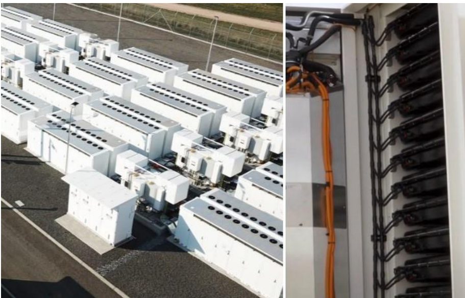
Figure 2 Example: Battery storage units and Lithium-ion battery pods
