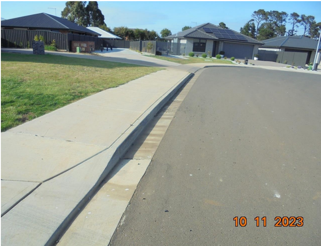
^Footpath outside adjoining property
