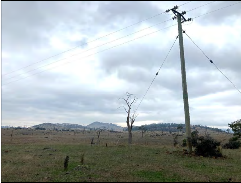
Image 9. Overhead powerlines and electric pole near proposed development site (taken at site assessment on 29/04/22).
