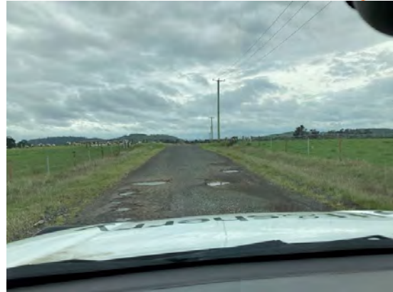
Figure 6: poor state of repair of Palmerston Substation Access Road
