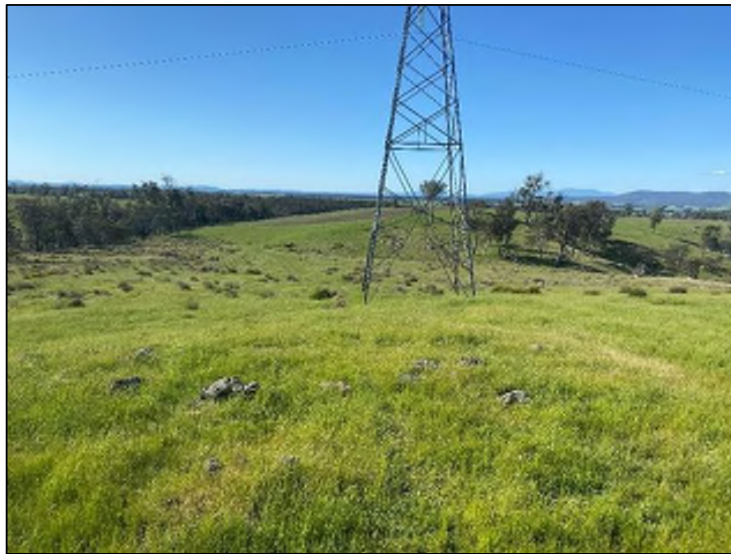
Figure 7: Existing transmission line in location of infrastructure zone.
