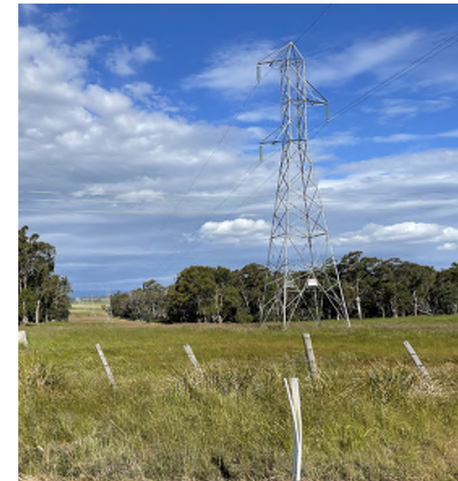
Image 06 - Transmission Line adjoining Macquarie Road
